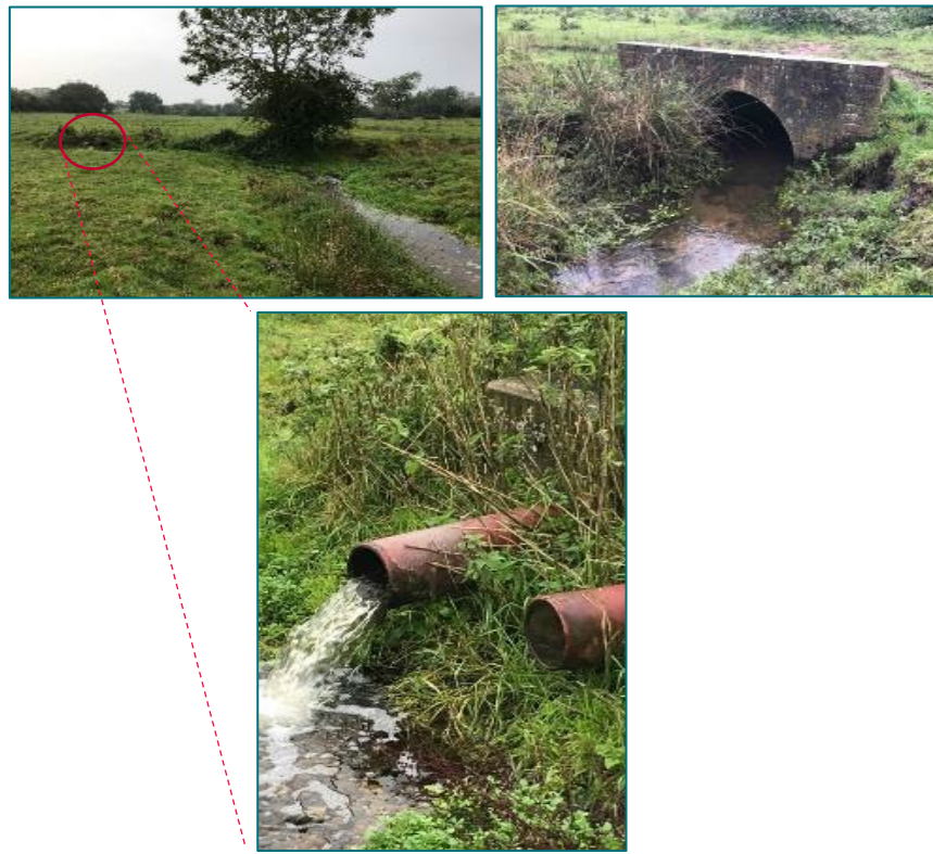
Plate 18.3.39: Outfall Pipes and Small Culvert
