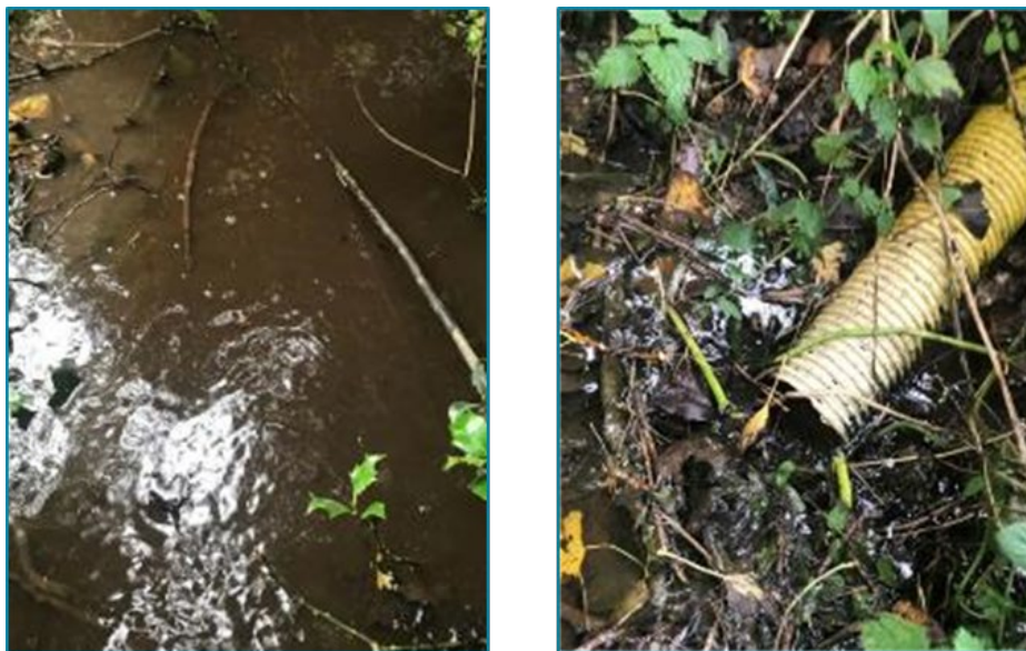
Plate 18.3.8: Silt Deposition and Outfall Pipe
